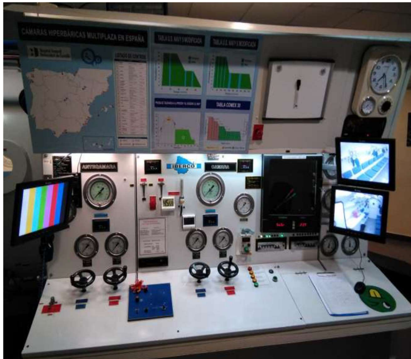
Panel de control
